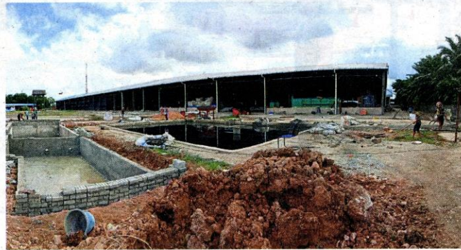
Filtration ponds under construction at the plastic processing factory in Batu 2, Sepang.
